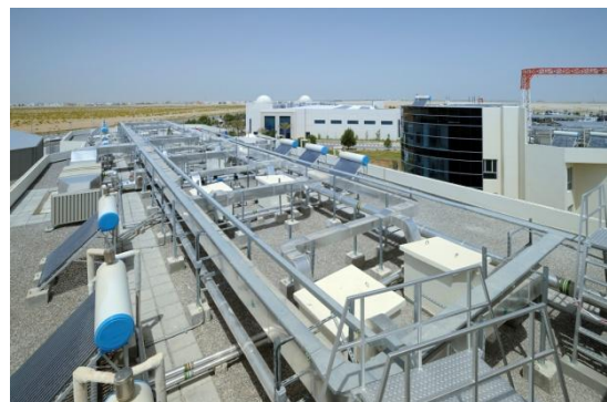
Image 2 – Solar water heaters & systems in place on roof
